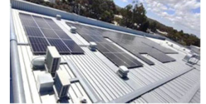
The solar power generation system at Jurlique's Adelaide factory
